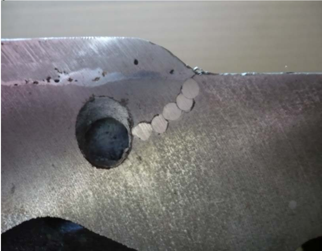
Second crack repaired 2009
